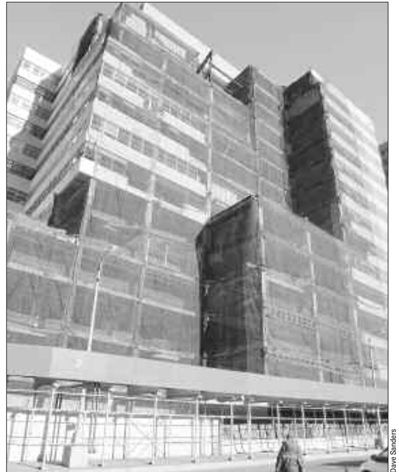
Fiterman Hall will be torn down – but a cleanup must come first.
