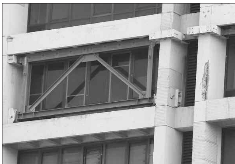
At right, rusting reinforcing rods force concrete to flake off. The braces, seen across the window, help hold the building up.
