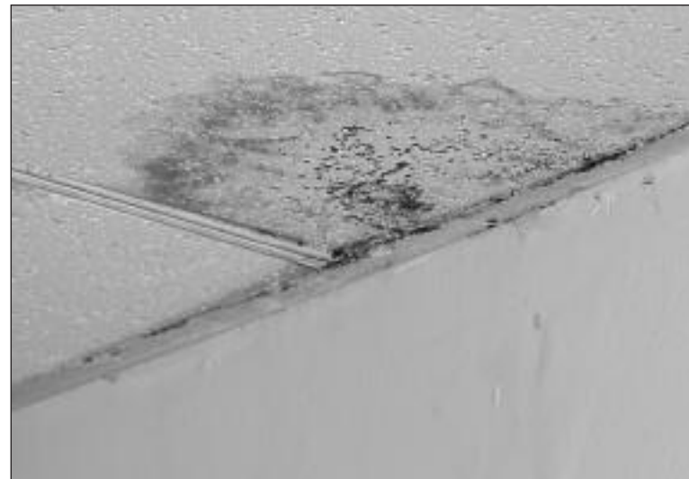
Mold found in some 75% of the buildings at CSI is causing respiratory problems for PSC members.
