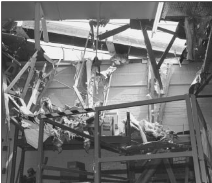
A crane collapse smashed a construction shed at Queens College in August 2001.
