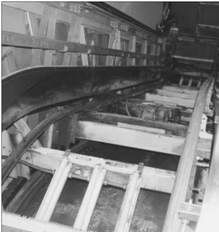
A common sight at BMCC: a broken escalator.
